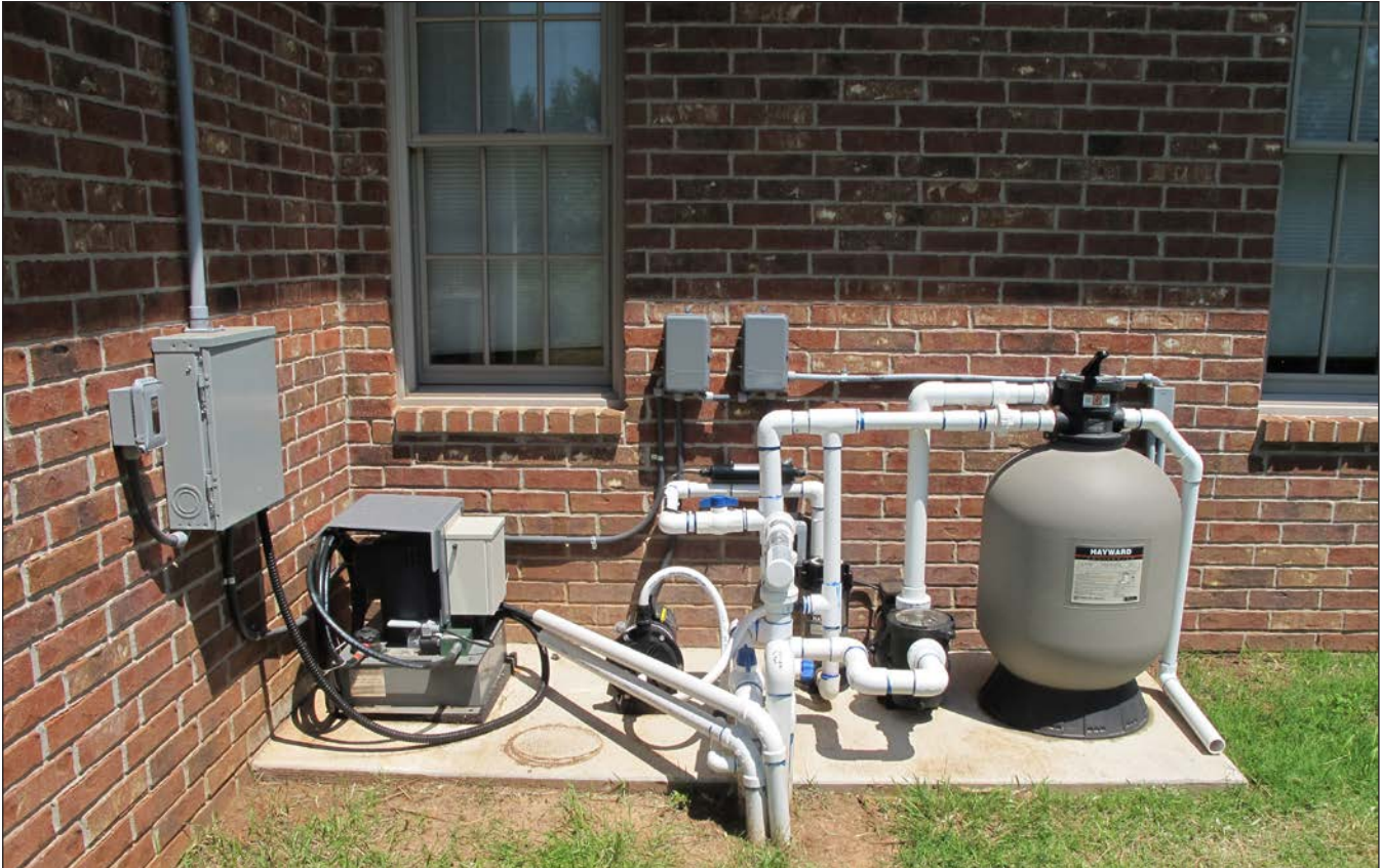
Figure 95: Place pool equipment in a safe area, sheltered from weather with enough space to maintain all equipment and eliminating any hazards.
