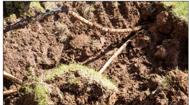
Figure 10: Be aware of underground services such as sprinklers and other private lines.
